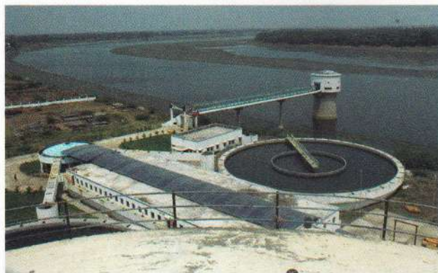
In 2002, Gujarat was the first State to plan clean tap water to every rural home
